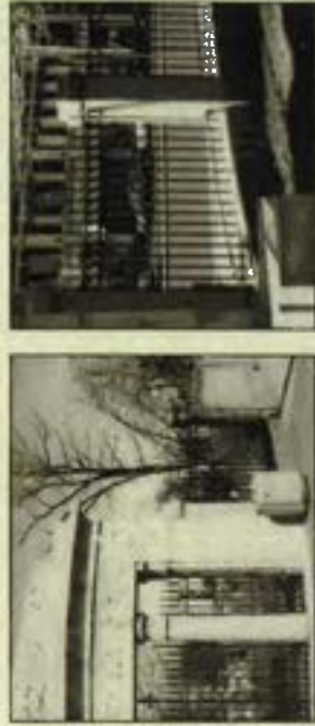
A section of the wall surrounding the Cornwheat North Burying Ground in Massachusetts was in a state of advanced deterioration. Roof, gutter, and foundation work were required to stabilize the structure. The area of wall between these parts was replaced with a new, decorative wall. The new wall was designed to be visually compatible with the original wall, allowing for visual access into the burial ground, where it was previously enclosed (photos: 1983 and Boston Photo)
