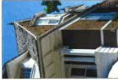
Wood shingles help to unify both walls and roofscape, creating visual feature as a background to Classical detail.
