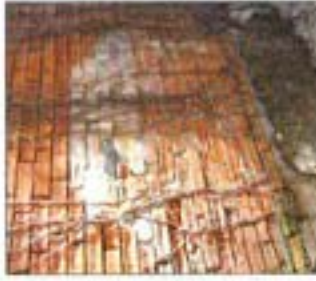
Great care is required to ensure that if cleaning is really required this is achieved using the gentlest means possible, and not using abrasive methods. In contrast to the care taken above, the brick surface below has been completely destroyed using abrasive cleaning methods.
