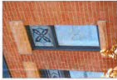
Matching the existing brick pattern or bond and the composition of the mortar help to ensure the integrity of the brick and stonework and consequently architectural character.
