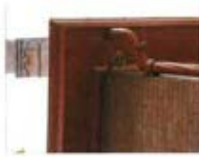
Gutters and downspouts may be a considered part of the building design.
