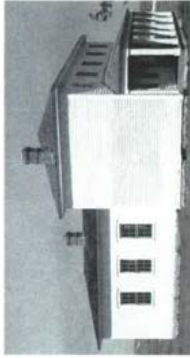
In a project at Fort Hays, Kansas, the wood frame officers' quarters were restored to the late 1860s—their period of significance. This included replacing a missing kitchen ell, chimney, porch columns, and cornice, and closing a later window opening in the main block. The building and others in the museum complex are used to interpret frontier history.
