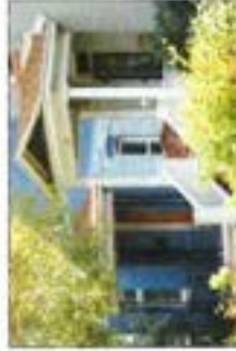
Wood columns and balustrades were commonly replaced with thin "wrought iron" railings and compromised the proportions and architectural integrity of the house.
