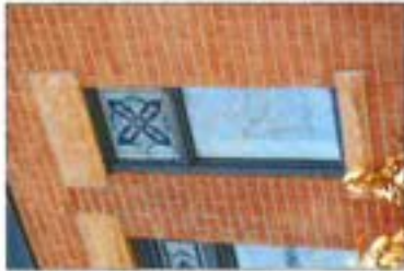
Matching the existing brick pattern to build and the composition of the mortar help to ensure the integrity of the brick and sashwork and consequently its architectural character.
