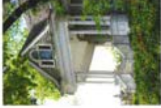
In this porch, grouped slender columns support an unobscure and the subtle above. These are key architectural features that should be preserved.
