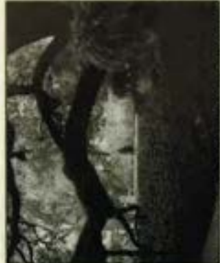
Fig. 10-10. A masonry wall in disrepair and being stabilized. (Author, 1997)
