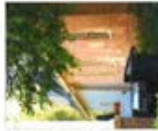
The rear addition respects the existing building by subordinate roof pitch, siding, and materials. The addition is designed to be subordinate in scale and character to the main building.
