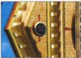
Brickwork, including the bond and mortar joint, width and profile, may be an essential component of the architectural character.
