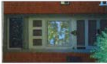
The design composition of the door, in this case with minimal glass transoms, is important to the architectural and historic integrity of the building.
