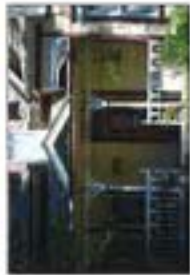
Repair original elements of the porch and consider retaining original features which have been lost.
