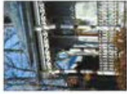
This porch reconstruction does not match the original porch.
