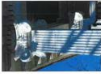
Periodic maintenance of painted surfaces and trim enhances the character of the building.
