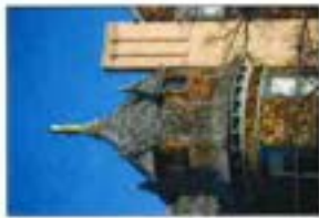
With the scale and work of many of the buildings in the district, roof materials can be a very important architectural characteristic.
