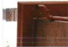
Gutters and downspouts may be a considered part of the building design.
