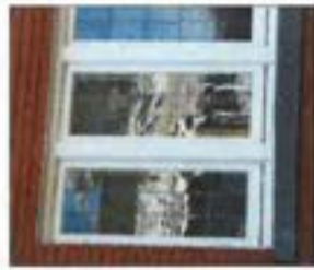
When a window is to be replaced, the new one should match the appearance of the original to the greatest extent possible.
