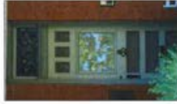
The design composition of the door, in this case with stained glass transoms, is important to the architectural and historic integrity of the building.
