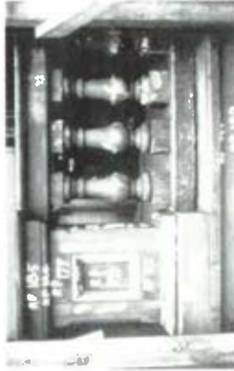
Portals of the small porch on an Italianate mansion were carefully numbered prior to Restoration. Some original elements were removed in place, while others had to be removed for repair, then reinstalled. Any elements too deteriorated to save was replaced with a new one replicated to match the original design. Photo: Morgan W. Phillips
