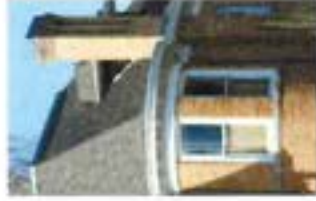
Apply shingles on the roof and replicate the existing material for the side and gable projections.
