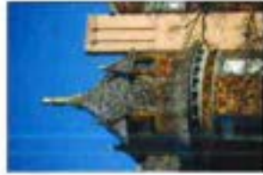
With the style and scale of many of the buildings in the district, roof materials can be a very important architectural characteristic.
