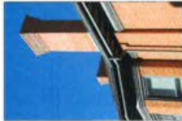
Variations in the brick texture and the pointing profile are used in this case to define the wall, the window bay and the chimneys.
