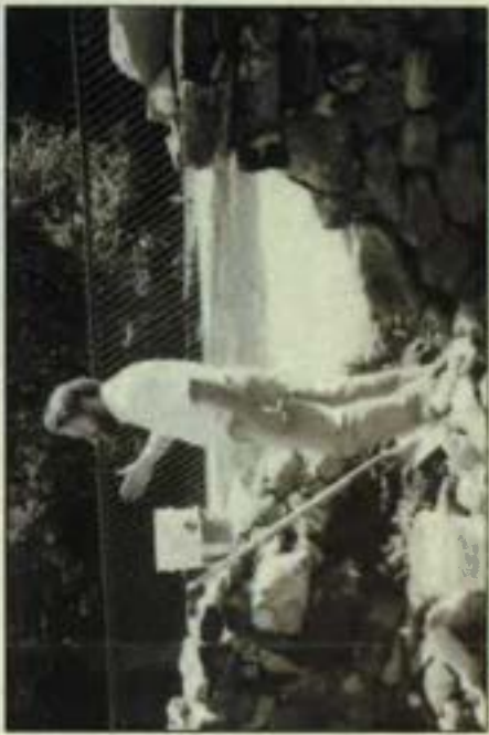
A section of a historic wall of the Hwayi Hall in Abano, Ohio, was in need of restoration. First, the fabric replacement of a section of the wall was undertaken using surviving stone and masonry that matched the old in form, size, and color. Compatible substitute material must also have been used. (Author, 1993)
