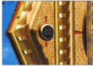
Brickwork, including the bond and mortar joint width and profile, may be an essential component of the architectural character.
