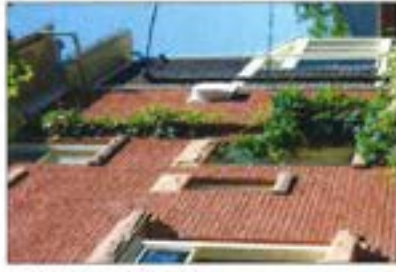
A new addition which is subordinate to the house and differentiated by height, materials, features/texture and window profiles and details.
