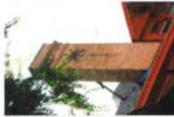
Seismic retrofit on one of the walls of a building through brick in the city.
