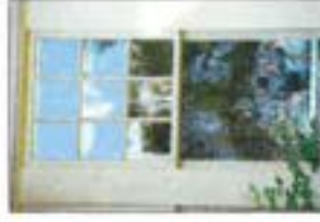
Windows help to define the design composition, style and historic integrity of a building.
