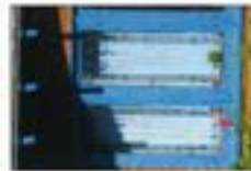
Historic window frames are well constructed and made from tough and durable wood. With minimum maintenance they will last as long as the building. Maintaining the glazing compound and sash and pane(s), with minimal maintenance of opening mechanism and sash rope(s), is usually all that is required when weather-stripping, and with the addition of a storm wedge, they will meet the energy efficiency or replacement requirements, rather than having to be completely replaced with a composite unit.
