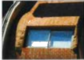
The appearance and integrity of the original masonry can be successfully maintained through appropriate repair.
