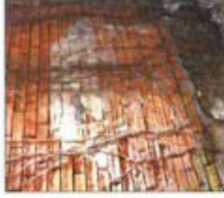
Great care is required to ensure that if cleaning is really required this is achieved using the gentlest means possible, and not using abrasive methods. In contrast to the case shown above, the brick surface below has been completely destroyed using abrasive cleaning methods.
