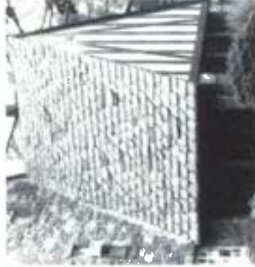
It is generally important to preserve materials that contribute to a building's historic character, such as the highly visible slate roof. In the event that repair and limited replacement are necessary, all new slate would need to match the old exactly. Photo: Jeffrey S. Lovine.
