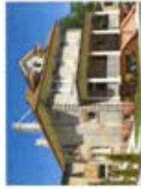
The Stranicek "Tough" Building, a wooden building built in 1906, has recently been retrofitted as part of an extensive rehabilitation.
