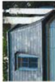
Natural slate eaves on the roof are the most desirable of historic materials. Carefully replicate only previous replacement of damaged individual shingles.
