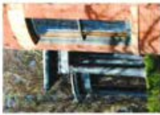
21. Never sash sills and pane at these heights are distinctive features that should be preserved.
