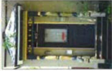
The design composition, materials, and detailing of the transoms contribute to the character of the building and its context.
