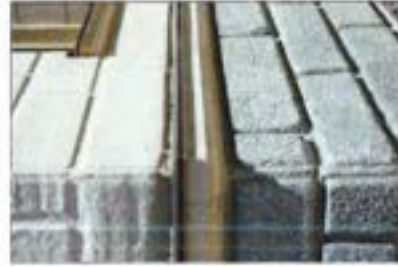
A new mortar profile demonstrates a sense of architectural time and history.
